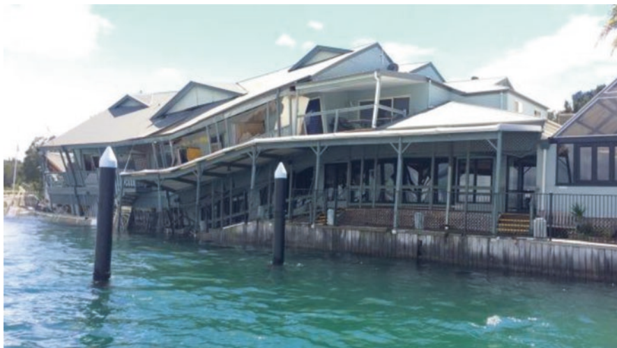
Fig. 10.30 Collapse of Swansea Channel foreshore building comprising restaurant, offices and residences on 8 February 2016 (Photo: Fire and Rescue NSW). The location is shown in Fig. 10.29. Particularly severe erosion has occurred along a revetment constructed to protect the western end of the airstrip. The revetment has attracted the channel thalweg, which has led to further scour both upstream and downstream, undermining the pile foundations of the building
